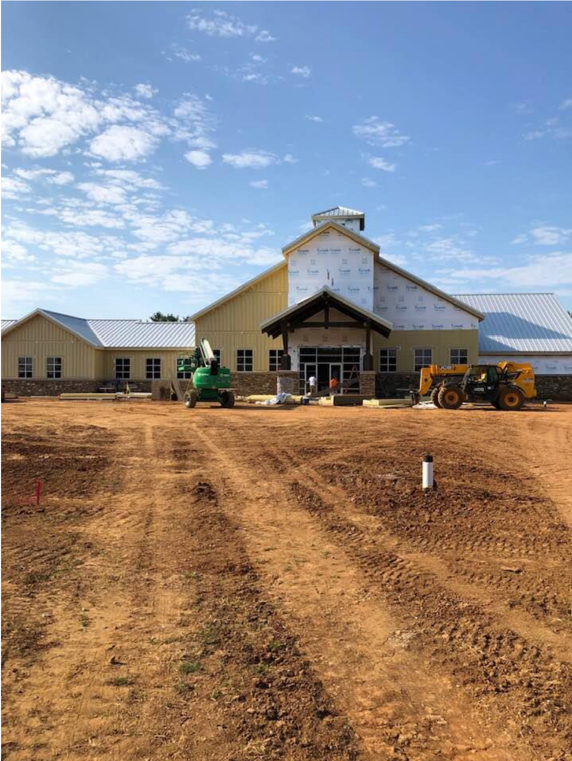
Work continues on the National Museum at the SCV Headquarters at Elm Springs in Tennessee
